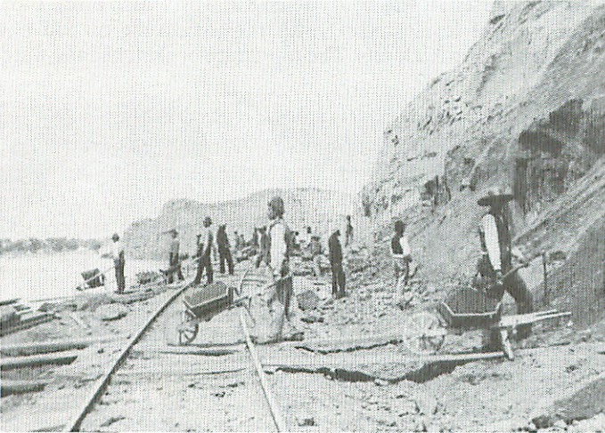
Northern Pacific work crew building grade and laying track in western North Dakota — 1880.
